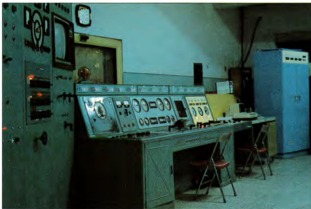
● Control room of FD-06 ● FD - 06控制室
